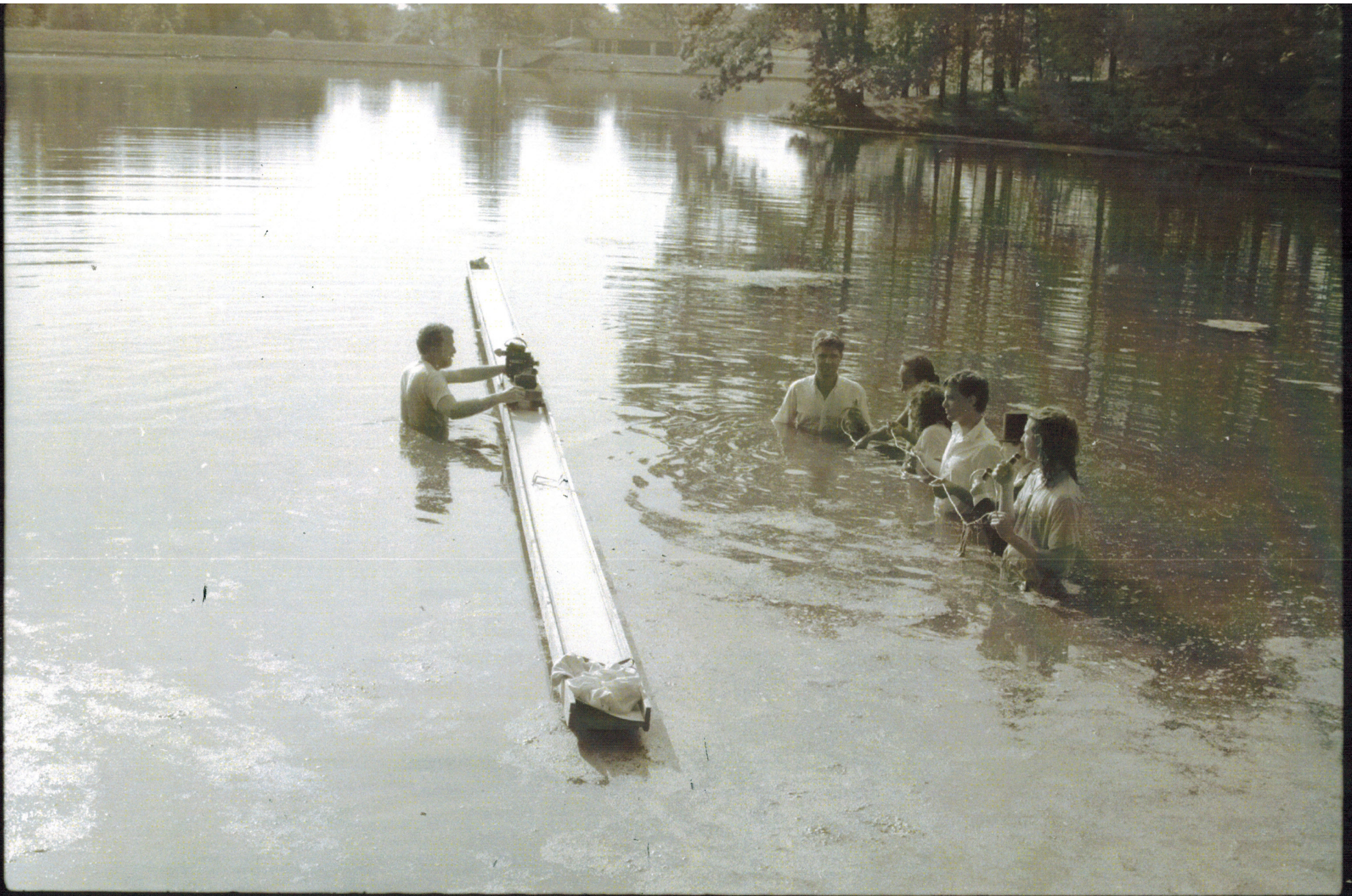
Another time I set up the platform on a lake which had a very soft muddy bottom. The tripods under it kept sinking into the muck.
